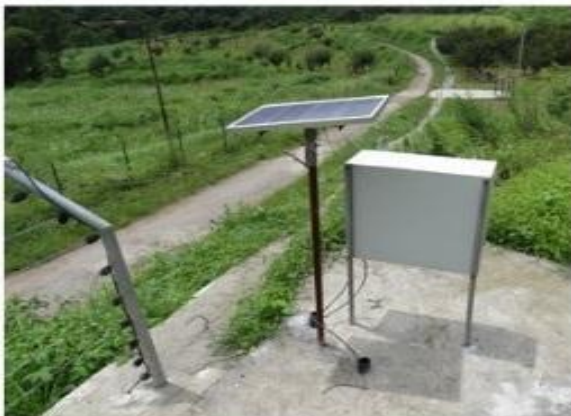
Solar Panel and control Unit
